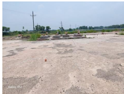
Figure 11: Pankhali yard no. 1, needs to be demolished (P-32)
